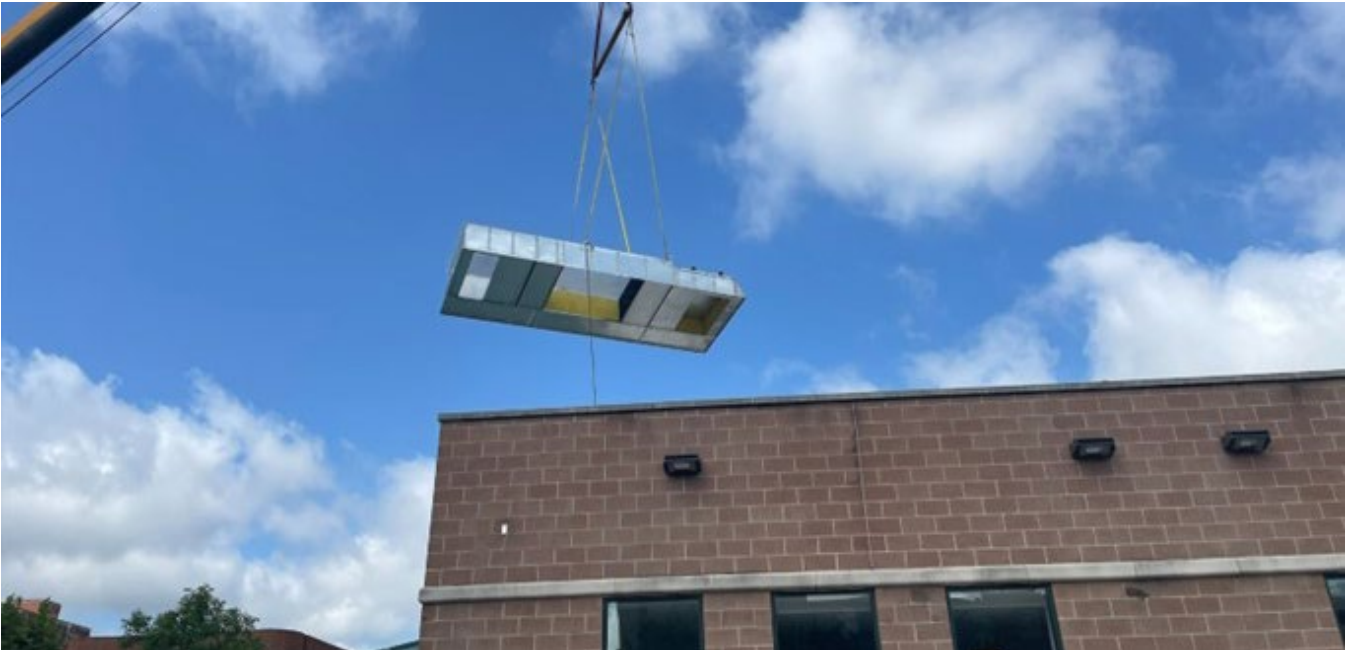
Installation of new roof top air handling unit at Provident Renal Dialysis Clinic
