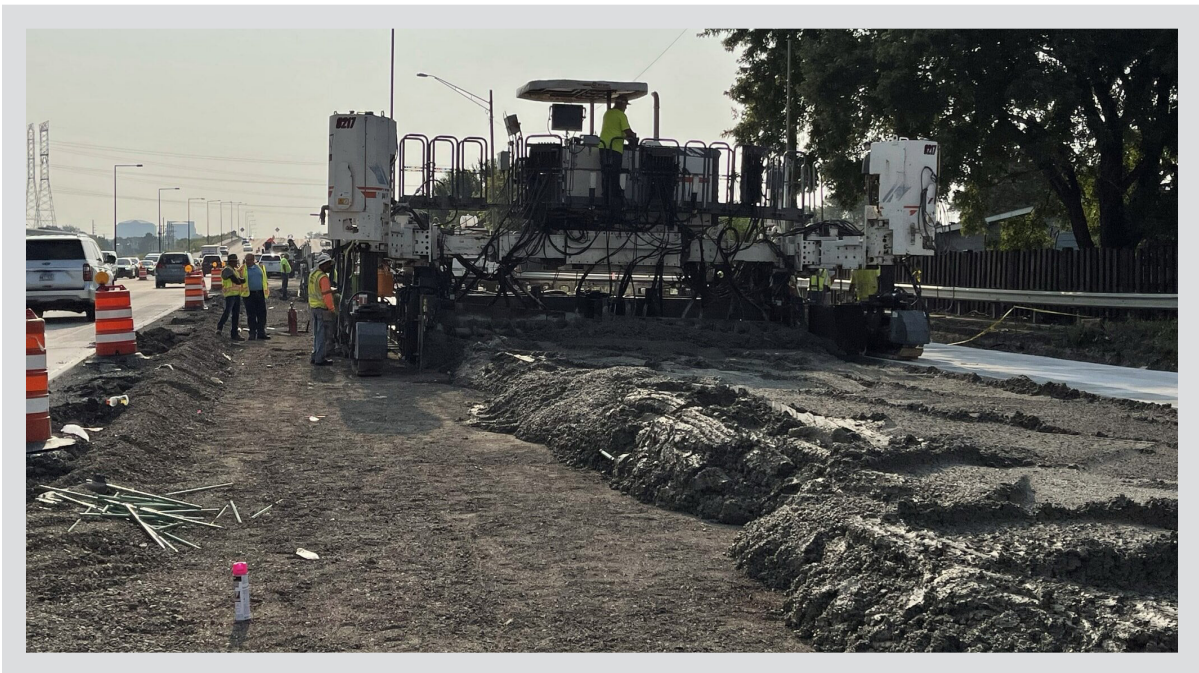
DoTH crews at work to repair and maintain asphalt and concrete pavement surfaces. Existing asphalt surface was removed by milling, full depth deteriorated pavement areas were removed, patched with concrete and roadway overlaid with a new asphalt surface.
