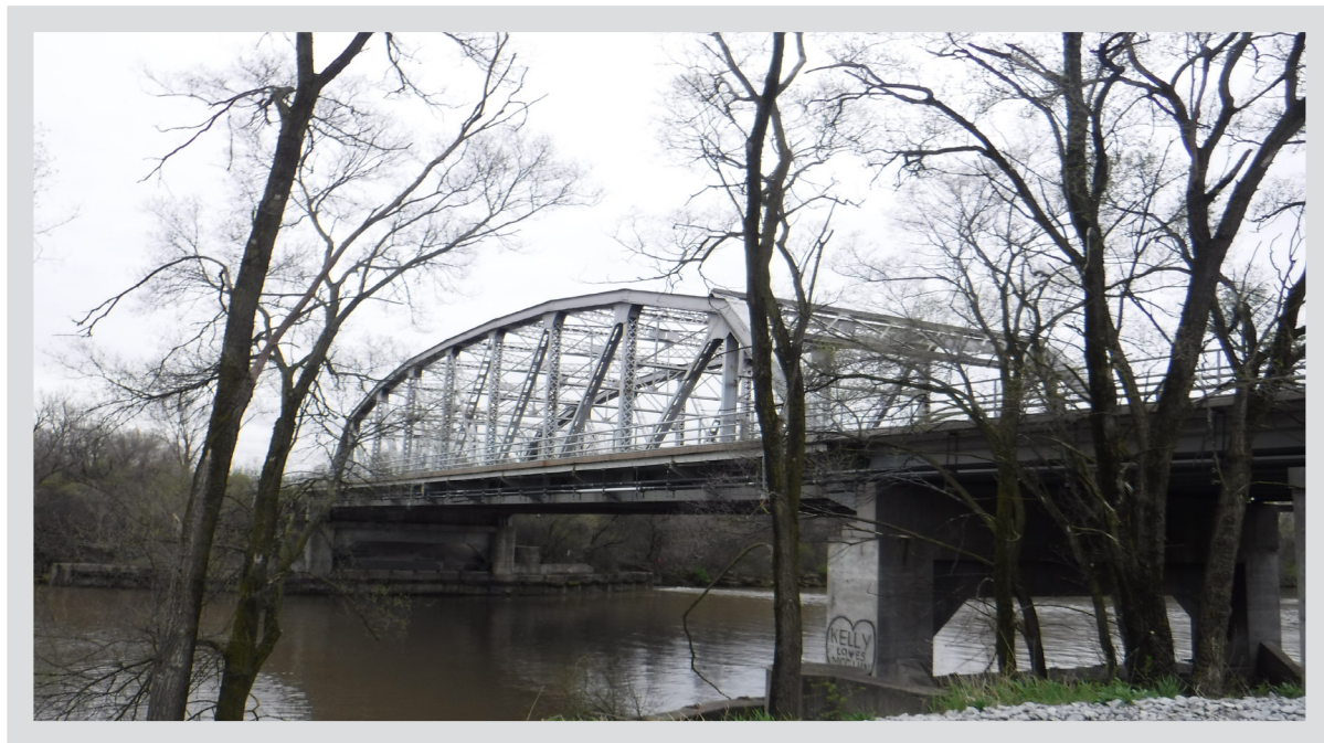
The truss bridges over the Cal Sag Channel are more than 85 years old and recent improvements extended the service life of the structure.
